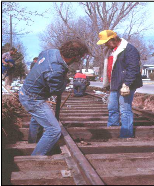
Les Batman assisting another volunteer connecting track panels at Shields St. After connecting new panels we lined, leveled and ballasted them by hand. Photo by Bill Kepner.
